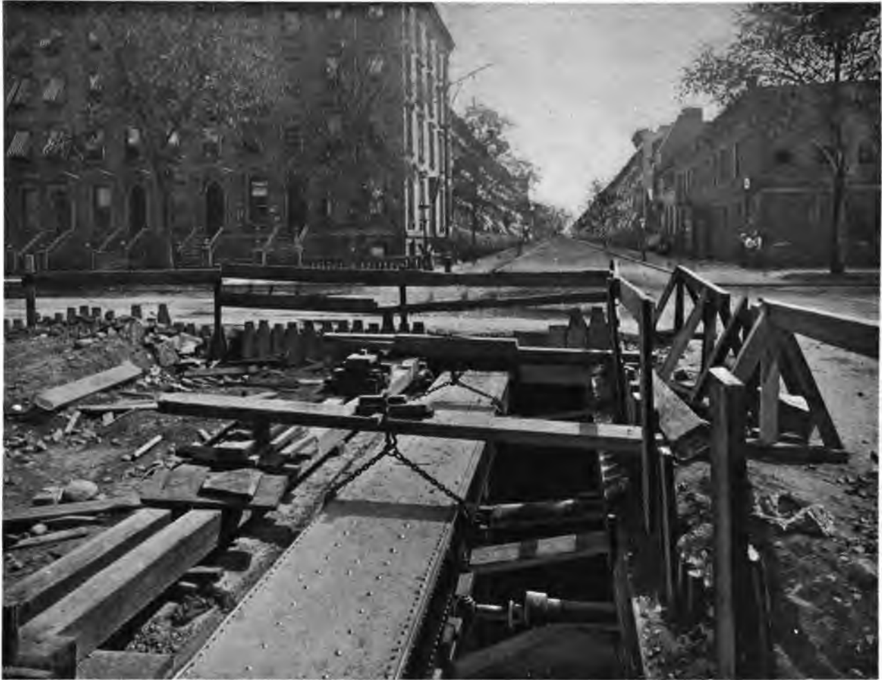
SPECIAL RIVETED RECTANGULAR WATER PIPE, OVER ROOF OF SUBWAY AT 126TH STREET AND LENOX AVENUE
